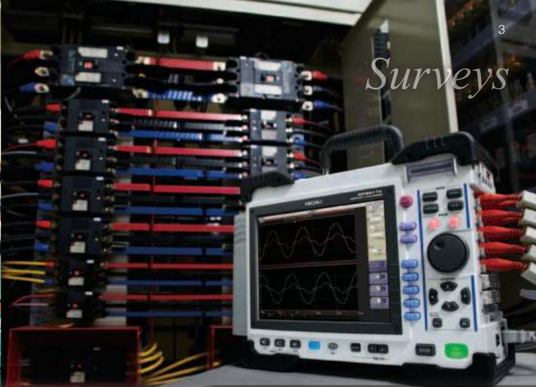
Power supply surveys for power equipment
